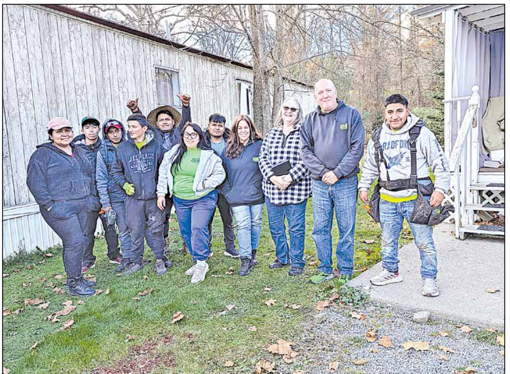
The Impact Project completed their 230th project at the home of Bonnie Evans in Sherburne, NY. A new roof was replaced with the support from 1st Choice Roofers and Renovations, Alpine Metal Roofing and Curtis Lumber Company. (Submitted photo)
