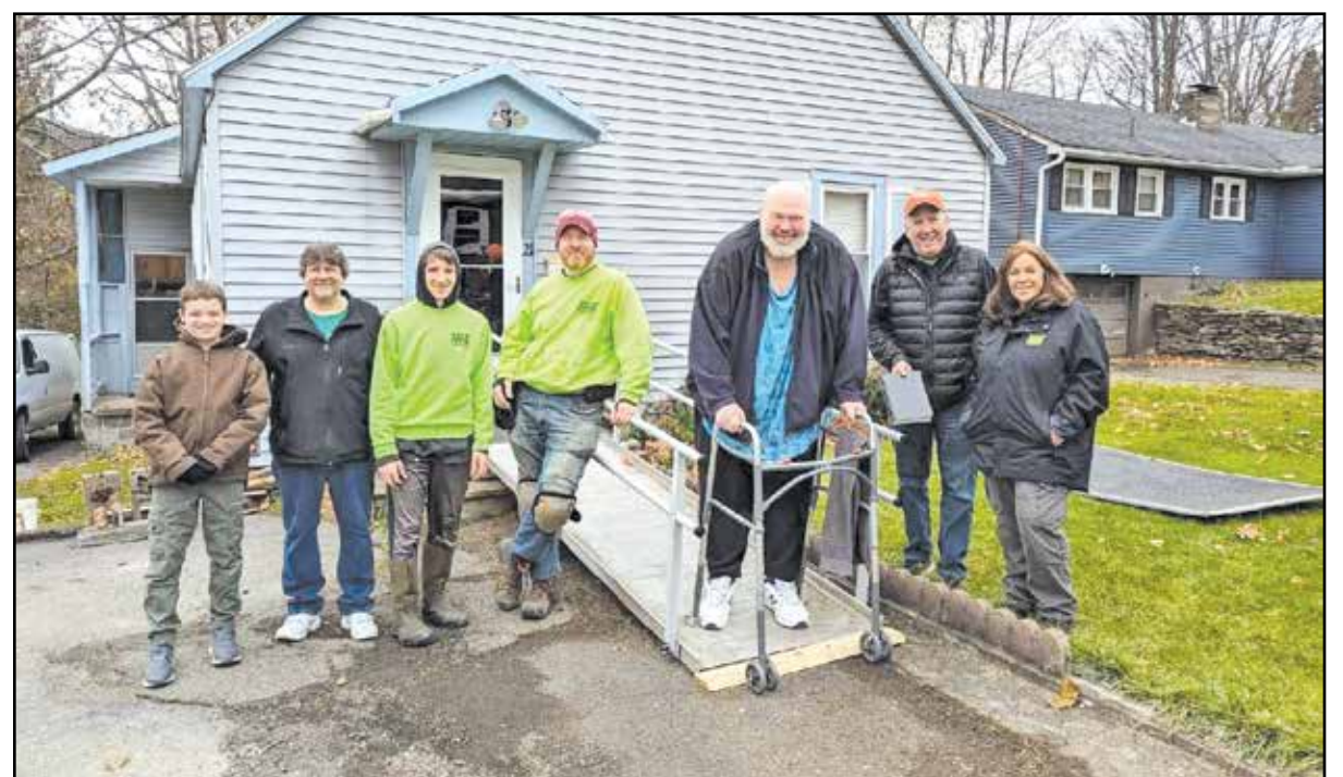
It was a double bubble day for Pat Rivenburg of Norwich when he received a handicap ramp and hot water tank plus plumbing repairs for the Impact Projects 186th and 18th projects. Support from Dave and Dean Westervelt and the Area Agency on Aging Chenango County was greatly appreciated. (Submitted photo)
